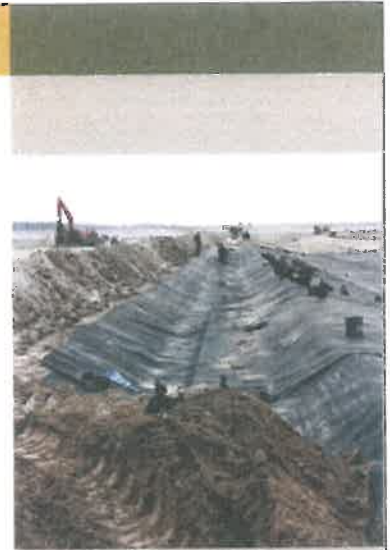
Crews install a geosynthetic membrane liner for an International Minerals & Chemical 192-acre landfill cell, the largest ever installed in the industry at that time.
