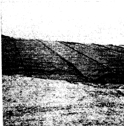
Cell WD-3 Northwest Sideslope Geonet/Geotextile Slippage Area After Repair View Toward West January 7, 1999
