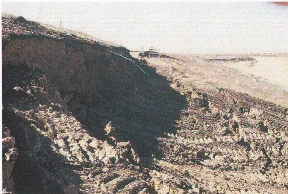
Exhibit TJFA 424-E, Excavation Slope Failure – Skyline MSW Landfill, 1999
