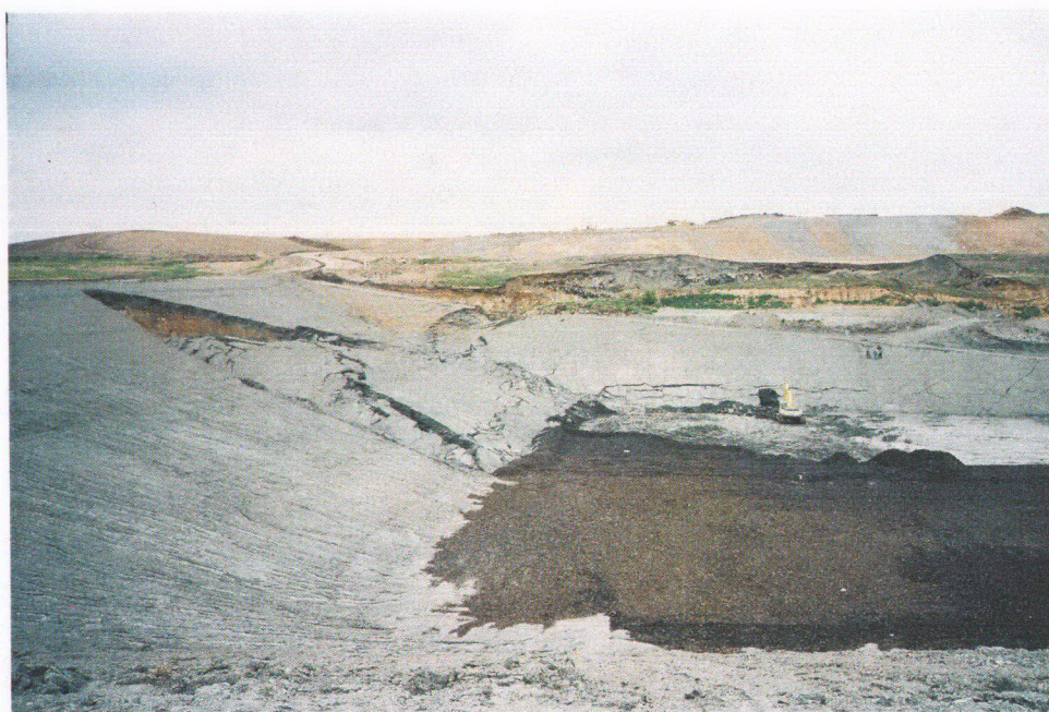
Exhibit TJFA 424-I, Excavation Slope Failure – City of Irving MSW Landfill, 1999
