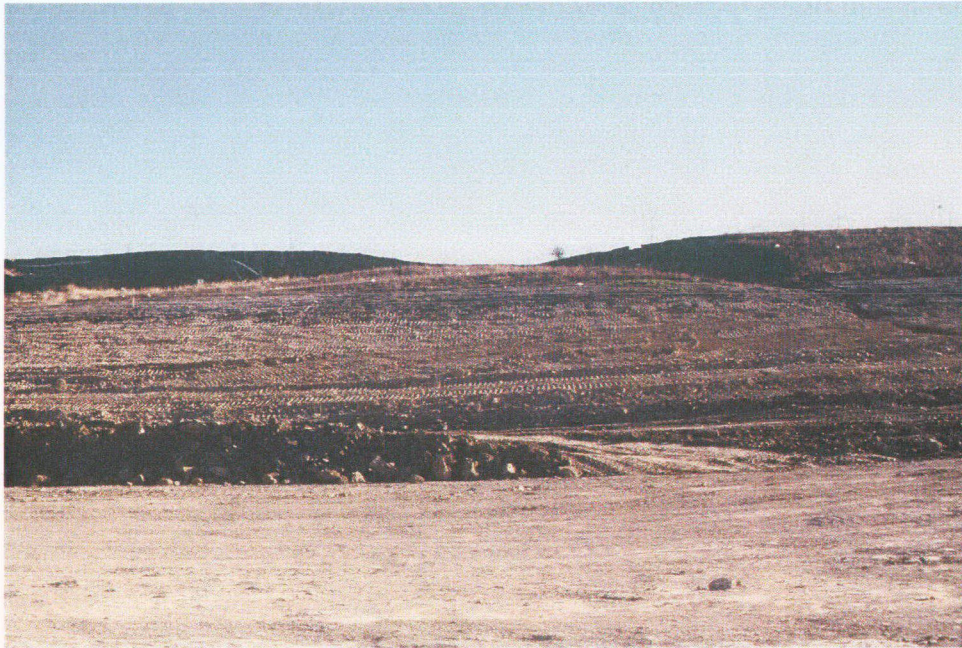
Exhibit TJFA 424-D, Excavation Slope Failure – Skyline MSW Landfill, 1999
