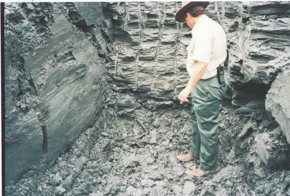
Exhibit TJFA 424-K, Excavation Slope Failure – City of Irving MSW Landfill, 1999
