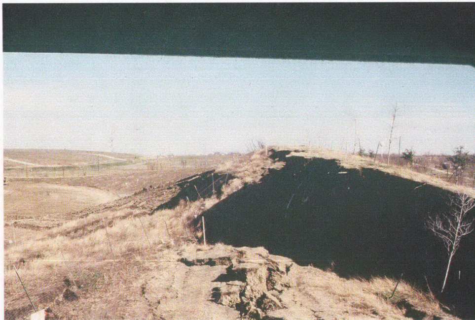
Exhibit TJFA 424-G, Excavation Slope Failure – Skyline MSW Landfill, 1999
