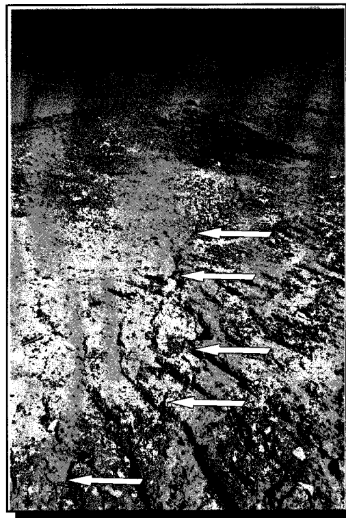
Figure 8-7 Expansion crack (marked by white arrows) that developed at the top of a slope of an Ohio landfill that had experienced a deep-seated translational failure involving RSL and unreinforced GCL. Contrast this with the damage at the toe of the same slope shown in Figure 8-8 .
